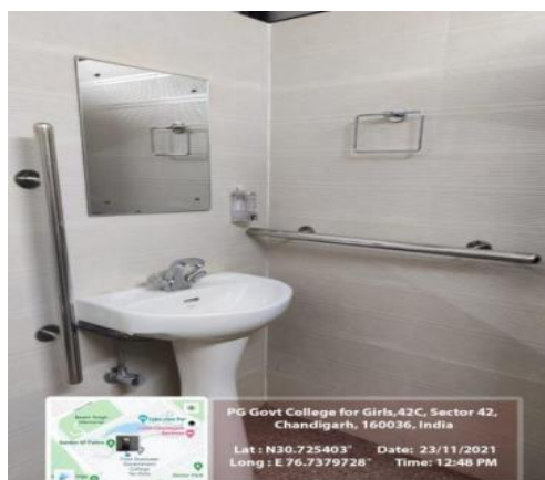
Disabled Friendly Washroom
